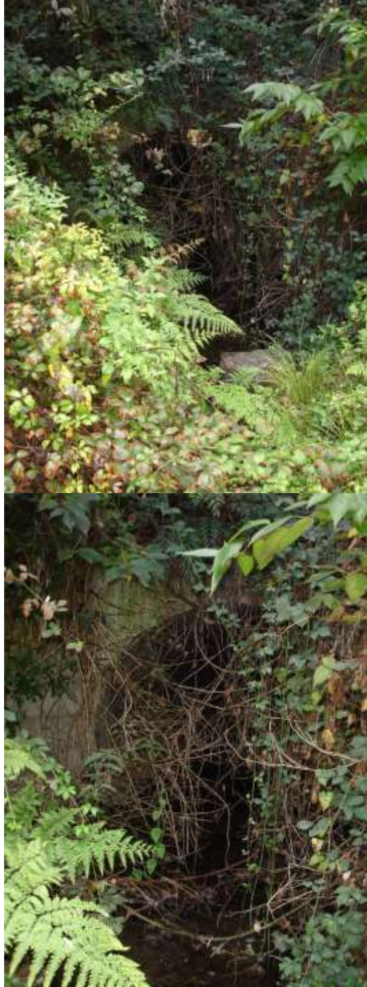
Figure 6: The culvert had a body of flowing water through it, making it impossible to scan with a GPR. The vegetation density and an uneven ground surface prevented GPR imaging.
