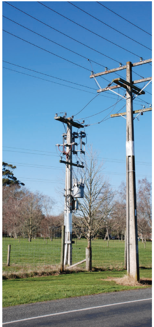
Tramway road transmission lines, Hamilton.
