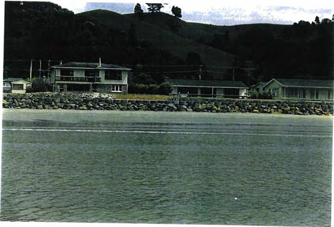
Plate 3: Rip rap in front of the middle and northern section of the sea wall.
