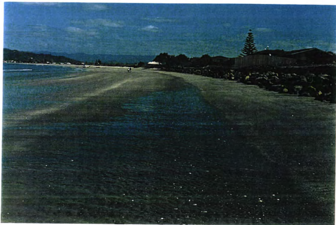
Plate 2: View from north to south along the wall showing "wetter" (muddier) intertidal zone in front of the northern section of wall as of October 2001.
